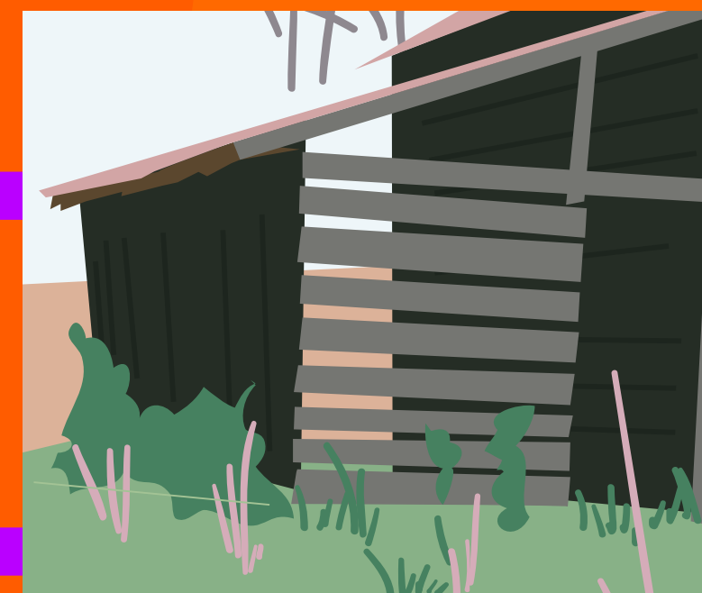
CLOSEUP OF WOOD LATS AND RUSTING ROOF
